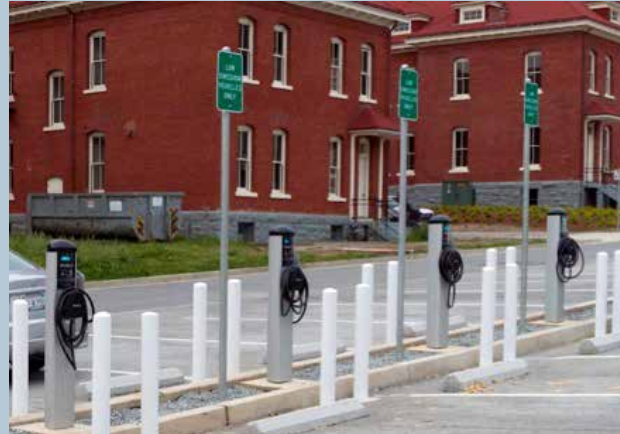
Parking lot with multiple charging stations
