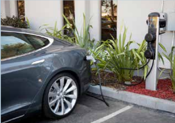
Car receiving electrical charge
