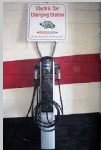
An electric car charging station for underground garage.
